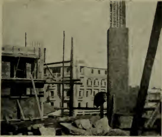
FIG. 5.—VIEW FROM FRONT OF FIRST FLOOR TOWARDS BACK WING UP TO SECOND-FLOOR LEVEL.
